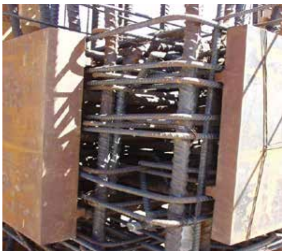
Fig. 3: Reinforcing bars must clear embed plates and studs by the clearance provided in Section 2.3.1 of ACI 117, and the SER must provide details showing how the clearance is to be maintained. This is particularly critical when the embeds have very thick plates (photo courtesy of Bruce Suprenant)
