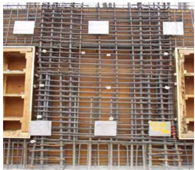
Fig. 5: A reinforced concrete wall with embeds and penetrations, shown prior to closure of the formwork. The embeds adjacent to the wall penetrations interfere with the vertical bars in the wall (photo courtesy of Bruce Suprenant)
